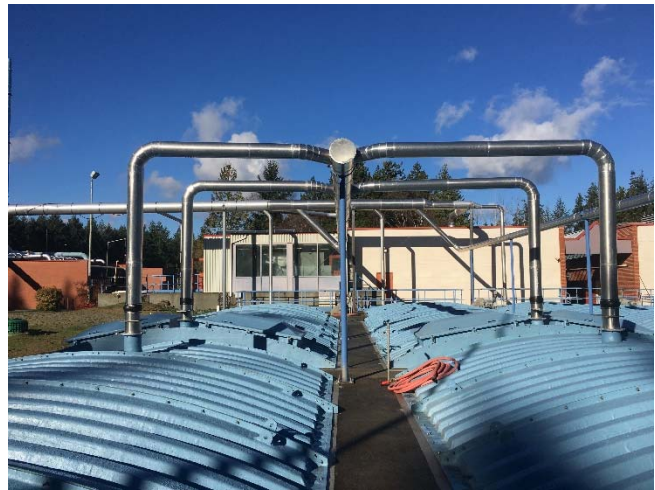
Photo 2- Primary clarifier covers and new ducting
