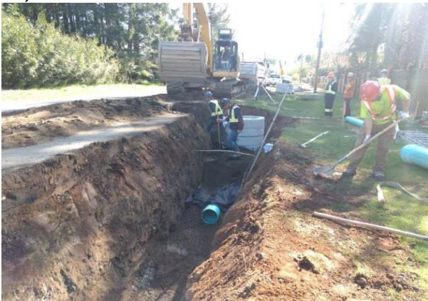
Photo 1- Sanitary pipe on Idiens Way
